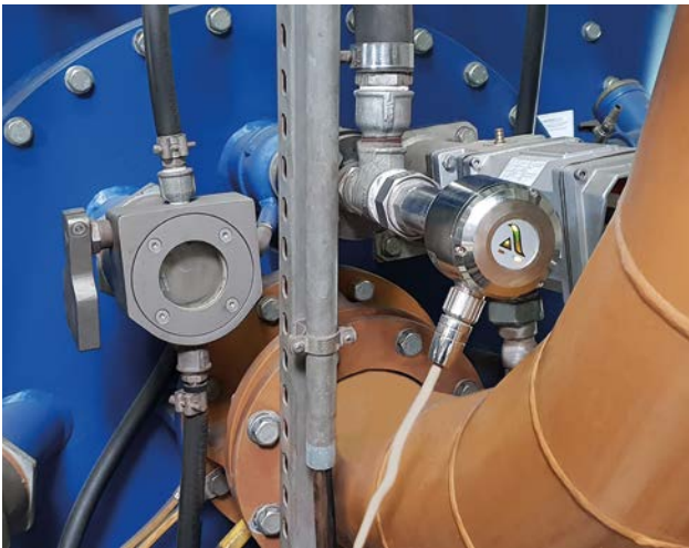
The LAMTEC F200K flame scanner in operation.
