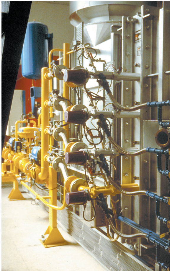
FlueFire system installed in a cogeneration plant
